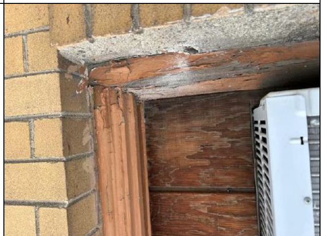
Brown Exterior Window Trim (LBP). (Photograph 6)
